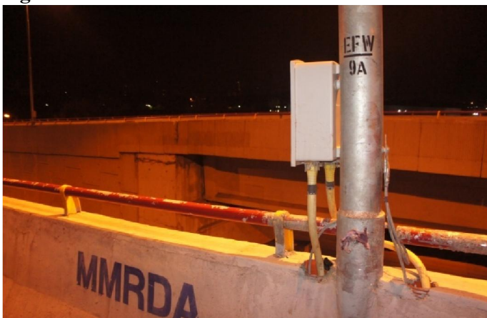
Fig.4:Pole on which accident occurred
